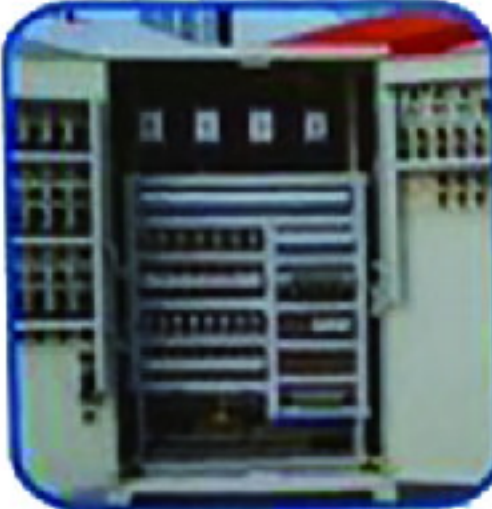
电柜特写 Electric Panel
